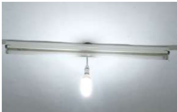
(e) Fluorescent still connected after being replaced with CFL.
