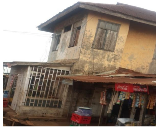
Plate 6 Mixed residential/commercial not maintained for over 50 years at Ona Ola road badly affected by weather Source: Authors field photograph (2017).
