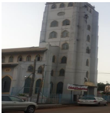
Plate 3 Cathedral church Ona Ola road completed for over 50 years Enjoys regular maintenance. Source: Authors field photograph (2017).
