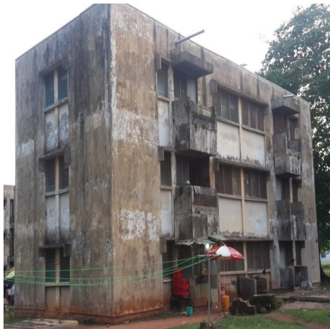
Plate 5, Residential building not maintained within 30 – 40 years at Federal Polytechnic Ilaro badly affected by weather. Source: Authors field photograph (2017).
