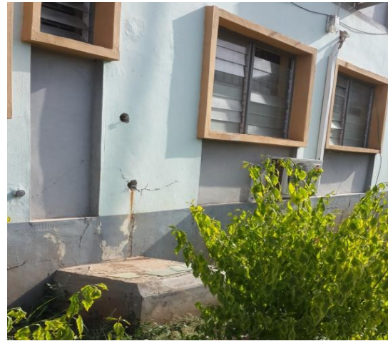
Plate 8, Administrative building completed within the last 10 years at Federal Polytechnic Ilaro fairly affected by weather
