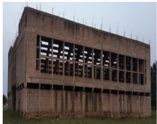
Plate 12 Sport centre Unplastered block wall abandoned for over 40 years at Federal Polytechnic Ilaro. Badly affected by weather.
