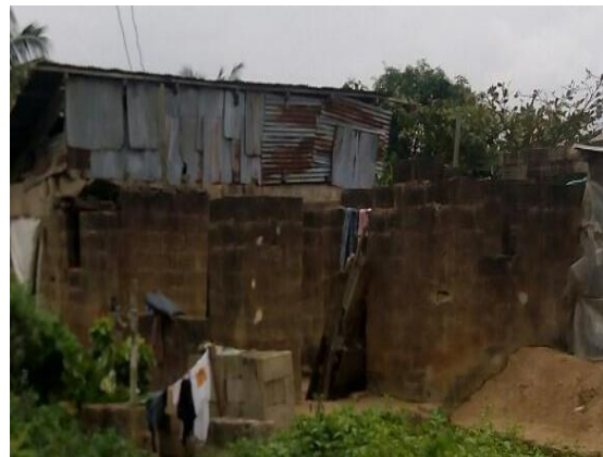
Plate2: Showing building condition
