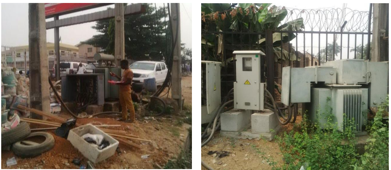
Figure 2. Data collection obtained from the transformer (Field Data, 2022).
