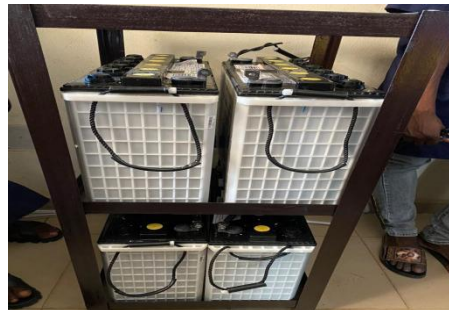
Fig 2: Pictorial view of 200AH (2units), 48V battery
