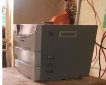
Fig 1: Pictorial view of 4KVA inverter
