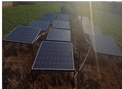
Fig 3: Pictorial view of solar panels (12units at 250W, 36V)
