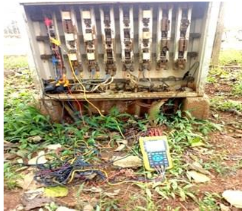
Figure 3. On-site data-acquisition equipment set-up
