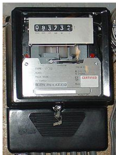
Figure 3: The Electromechanical Meters.
