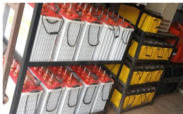
Fig. 4. Various types of battery in a typical solar system installation.
