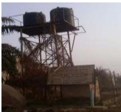
Fig. 1. A moribund solar-powered borehole in Akure Ondo State [12].
