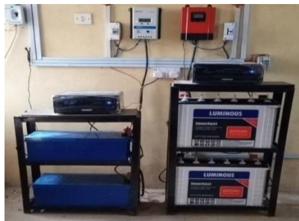
Fig. 5. Solar system installation showing solar controller, batteries, inverter, and DC circuit breaker installation for protection.
