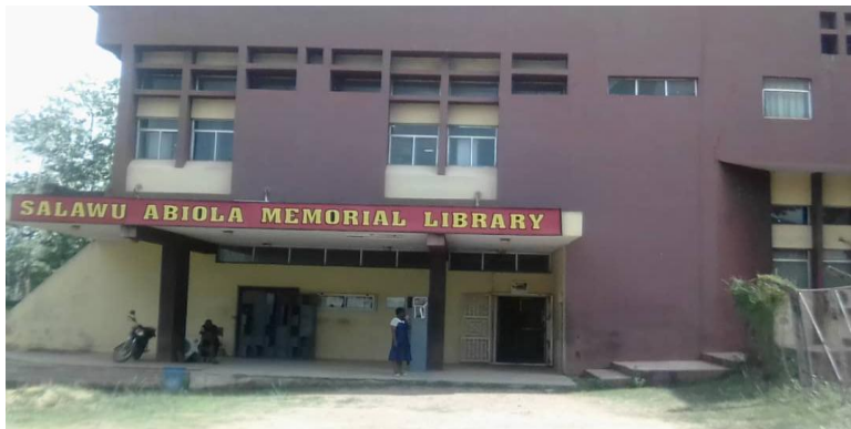
Fig. 2 Approach view of Salawu Abiola Memorial Library, MAPOLY, Abeokuta, Ogun State, Nigeria; showing imminent need for total restoration towards achieving sustainability
